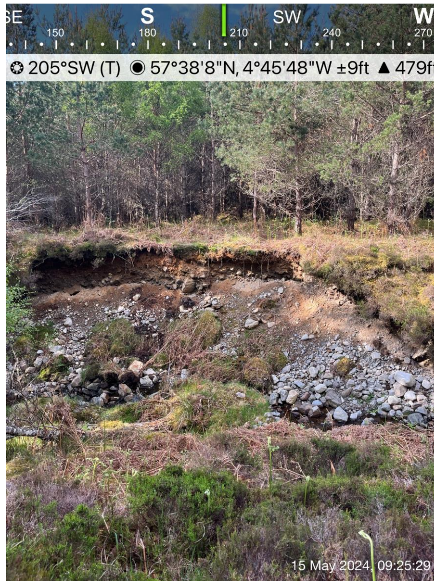
Photograph 8: View southwest towards an exposed eroded bank within the Site
